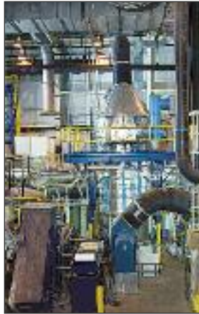
The WESP installed on Mayo Clinic's incinerator.
